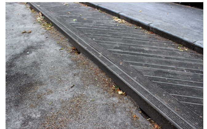
Rat holes under timber decking
