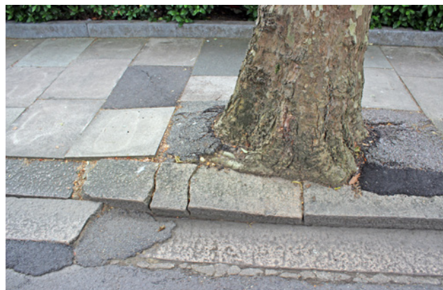
Surfaces in need of repair
