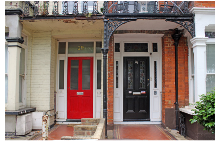
Recessed pair of porches with flat arched entrances and remaining fragments of original iron balcony and supporting structure (Nos.29 and 31)
