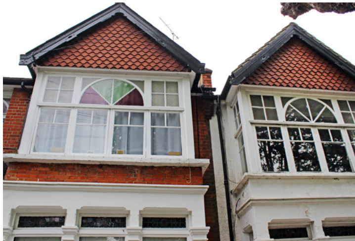
Detail of Edwardian detailing on houses to the east end of the terrace with distinctive glazing bar design
